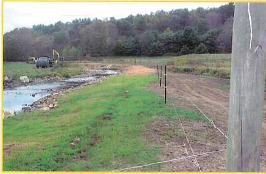
Figure 13. Electric fence installation along the outside edge of newly created riparian zone.
