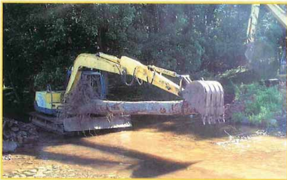
Figure 4. Excavator moving into position to install a rootwad into the streambank for flow deflection and fish habitat purposes.
