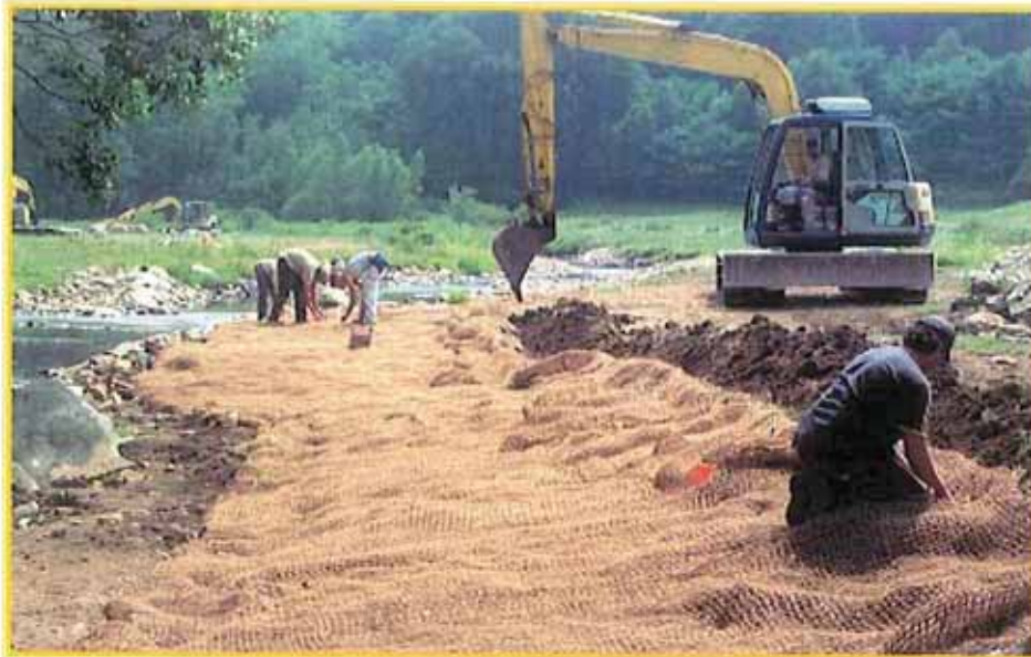
Figure 3. Installation of coir erosion control blanket along the newly created bankfull bench.
