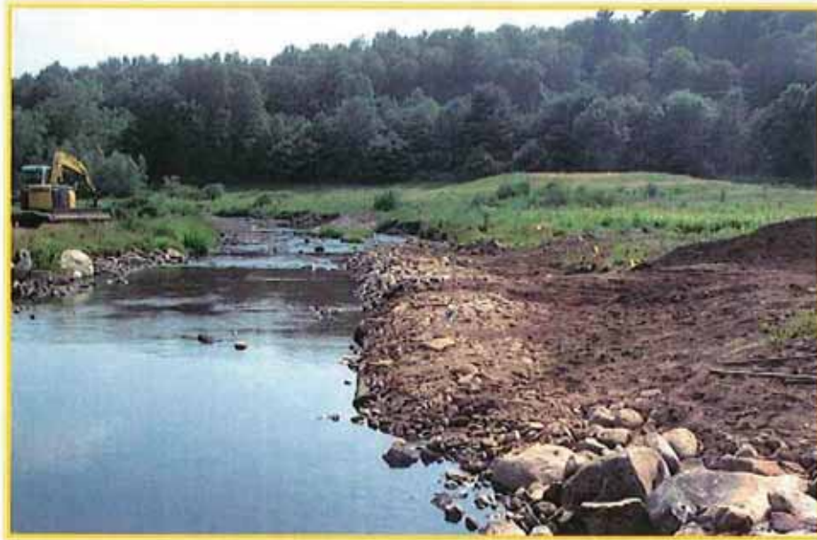
Figure 9. Photograph showing final grading, reduction in channel width and creation of bankfull bench.
