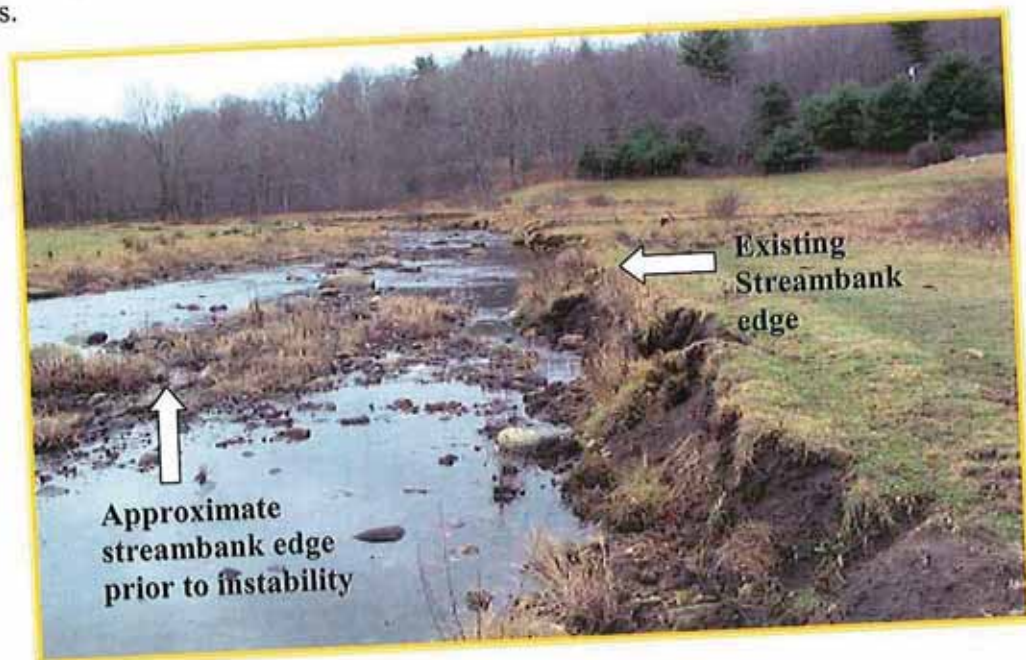
Figure 3. Example of streambank erosion and stream widening along Mount Hope River prior to restoration.
