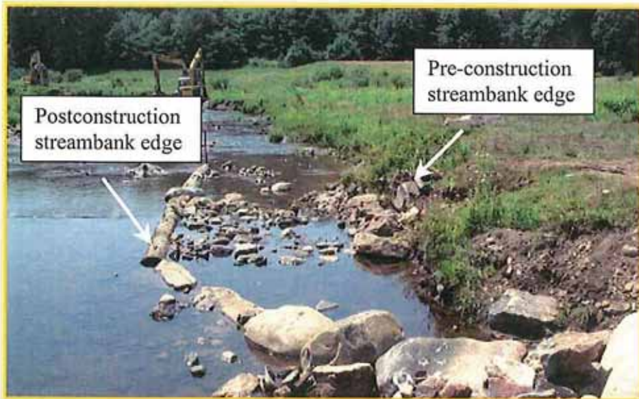
Figure 8. Photograph comparing preconstruction streambank edge and area of channel that will be filled to create the bankfull bench.
