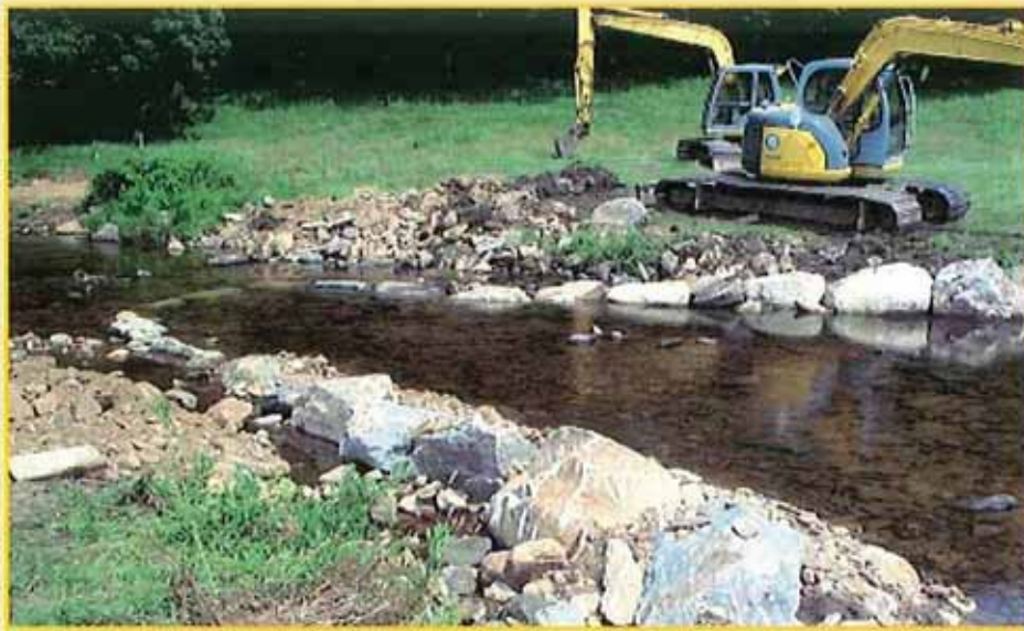
Figure 1. Completed construction of cross vane at station 12 + 10 immediately below the upstream cattle crossing.
